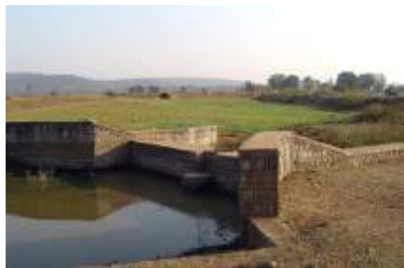
One of the two check dams
